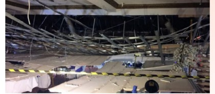
Figure 3. Inadequate fixings. Picture credit: West Midlands Ambulance Service
