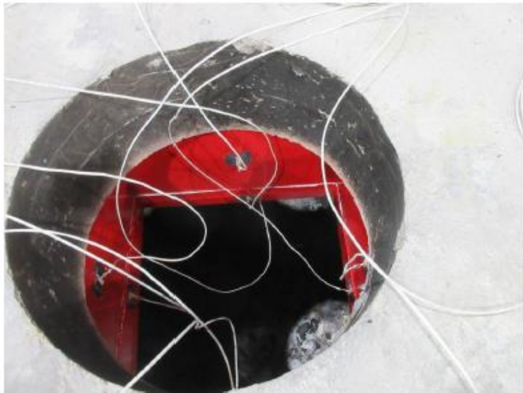
Photo 8. Chute viewed from Non-fireside (with installation of thermocouple for information only).
